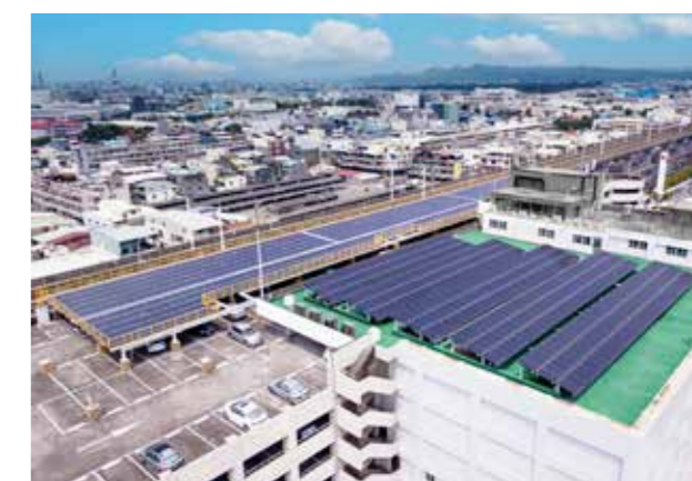
..... Solar Power Panels of Renwu Plant in Kaohsiung
